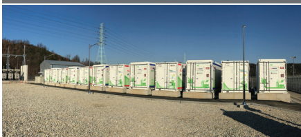
KEPCO Shingeryong substation
